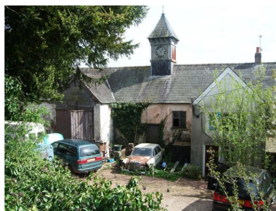
Fig.51 Court Farm. This range with its eye catching clock tower is unfortunately in a poor state of repair
